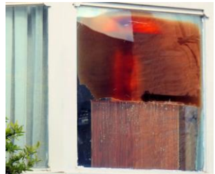
71 Hobden Window Fail Photograph £180
